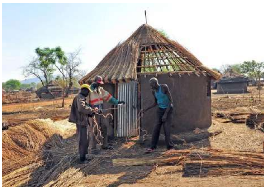
Construction Group A1 renovating a tukul's roof in Nyumanzi (Photo Credit: The Lutheran World Federation (LWF))
